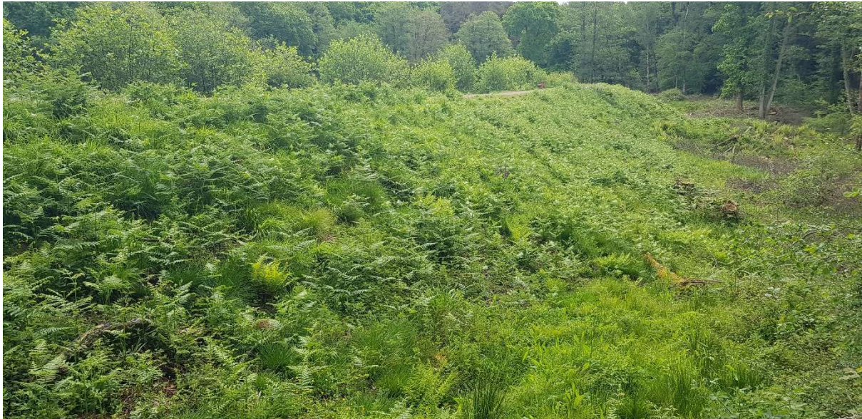
Photograph 5: Embankment downstream face with significant vegetation growth
