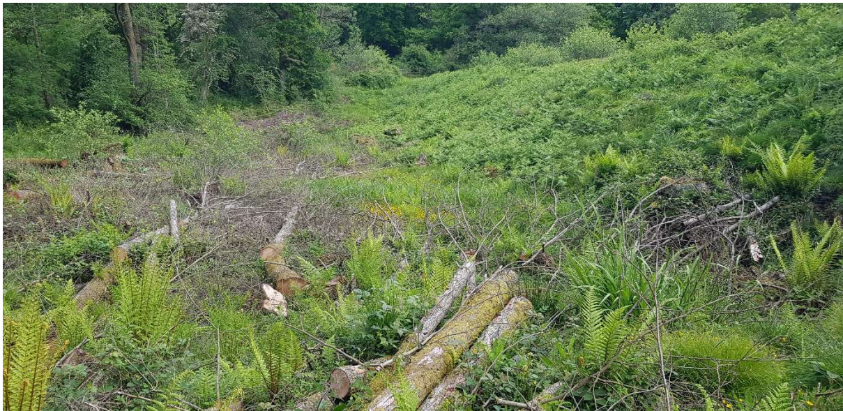
Photograph 6: Embankment downstream toe with significant vegetation growth and cut tree logs
