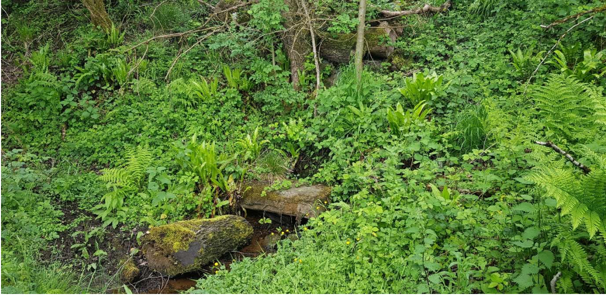
Photograph 9: Exit to culvert passing under B4234 and discharging to area downstream of embankment right mitre
