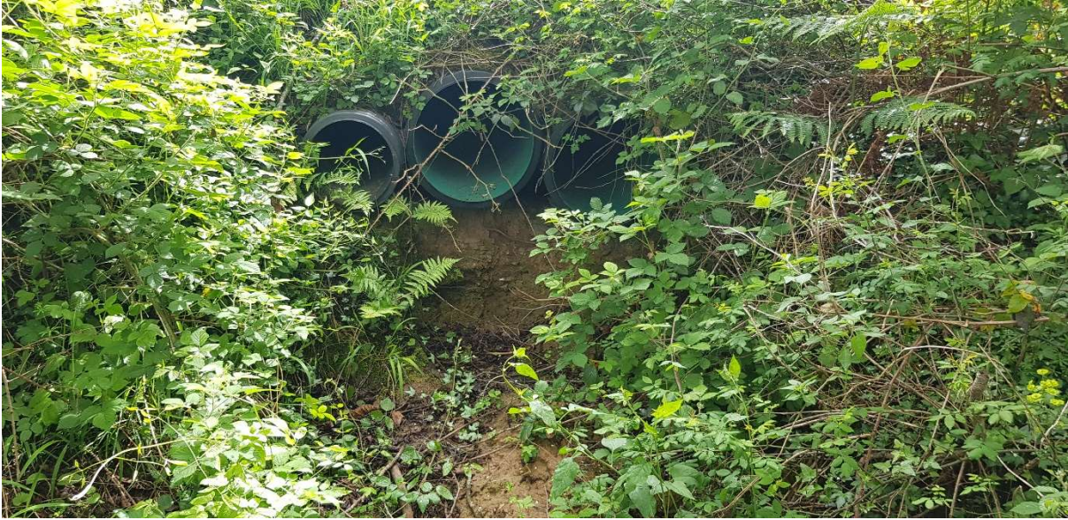
Photograph 17: Culverts under road embankment near to left abutment bringing flows from eastern catchment into reservoir during high rainfall
