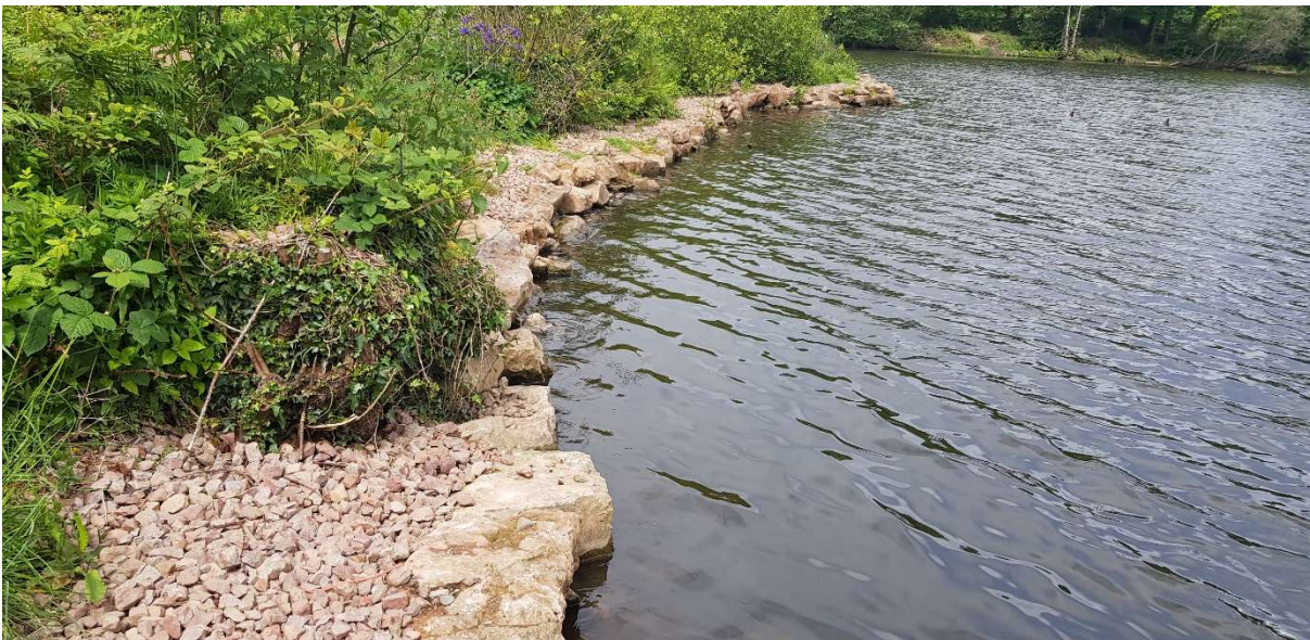
Photograph 2: Embankment upstream face with stone block protection and vegetation growth
